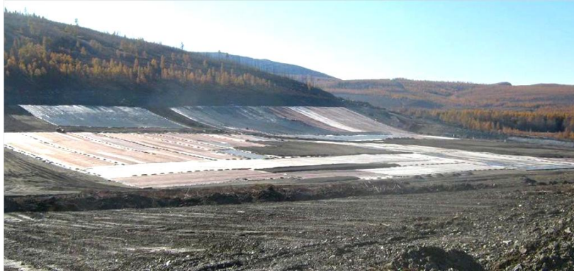
Figure 1 – The Use of Geosynthetic Screens in the Development of industrial waste storage
