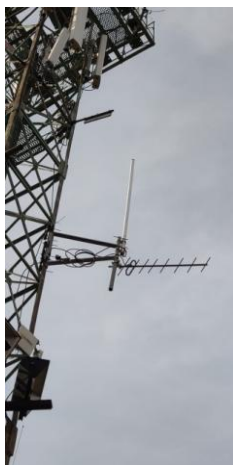
Figure 1 – VHF antennas of the BSDC transmitting complex on the Control's room antenna mast
